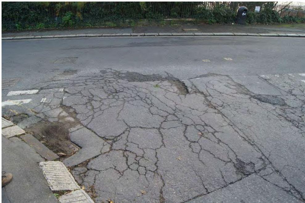
Photo 9. Cracks and silted up drain visible in the road forming the junction between West Hill and Archery Road.
