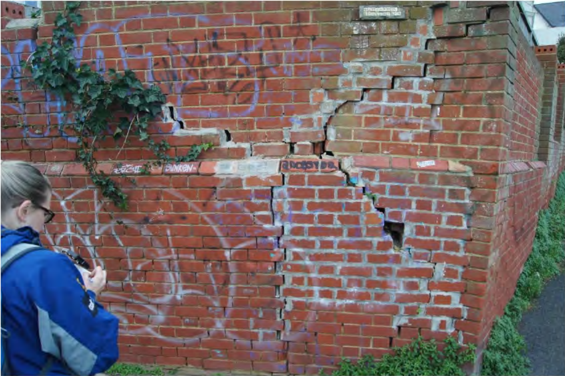
Photo 3. Southern face of Wall B showing extensive cracking and significant horizontal displacement of bricks.
