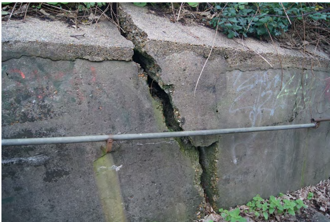
Photo 4. Large crack on Wall C. Broken railing can be seen on the right side of the photograph.
