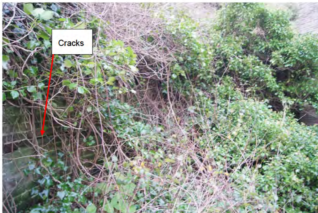
Photo 6. Wall E exhibiting some cracking.
