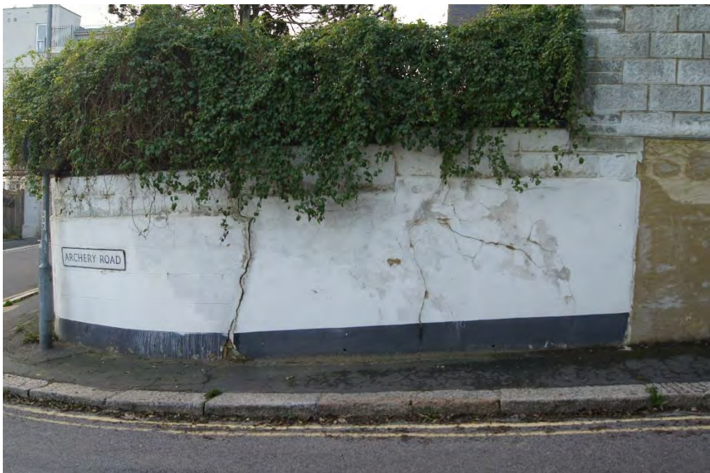
Photo 10. Cracks visible in the wall forming the junction between West Hill and Archery Road.
