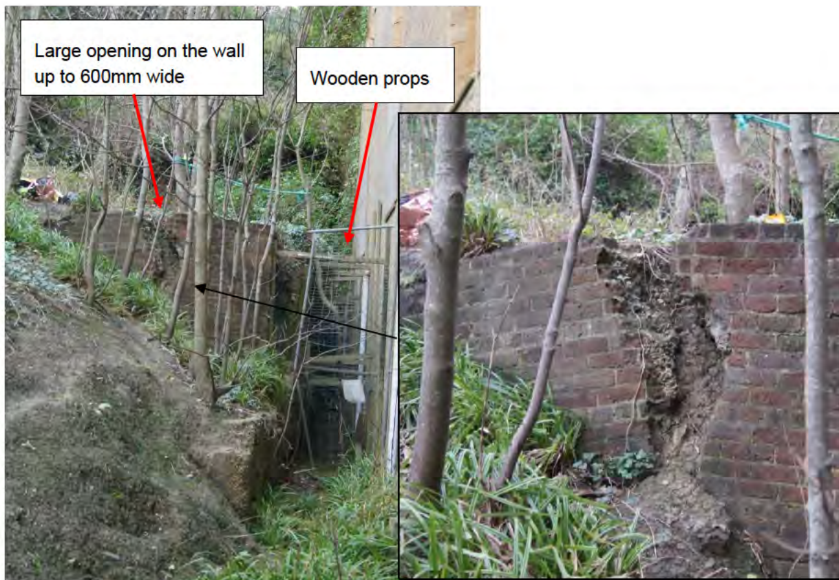
Photo 5. Wall D leaning towards the church.
