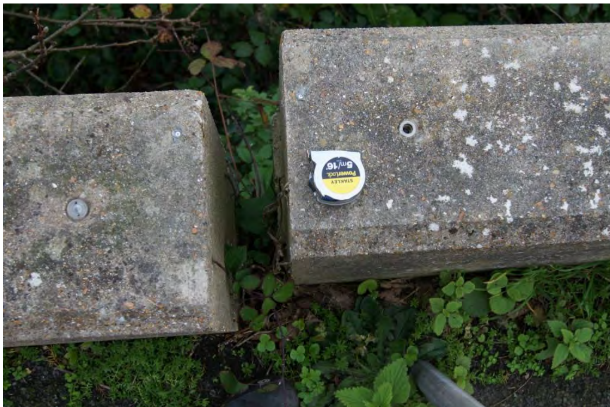
Photo 1. Wall A. Joint opening and rotating with a displacement of 100mm to the south.
