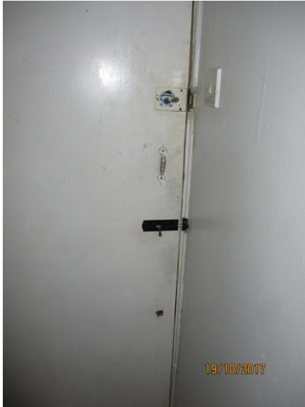
Lock missing to flat entrance door
