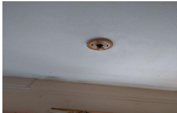
Smoke Detection System
