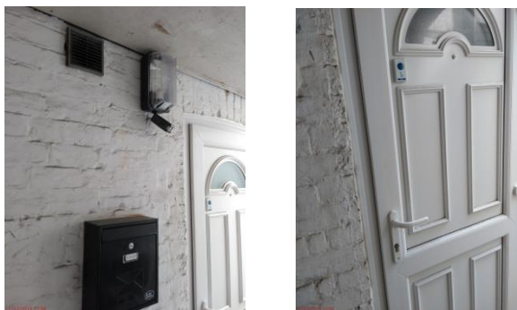
The new security light and UPVC front door
