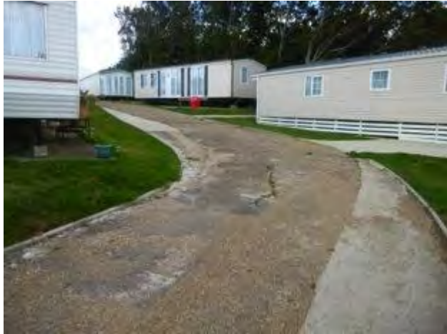
Road requiring repair
