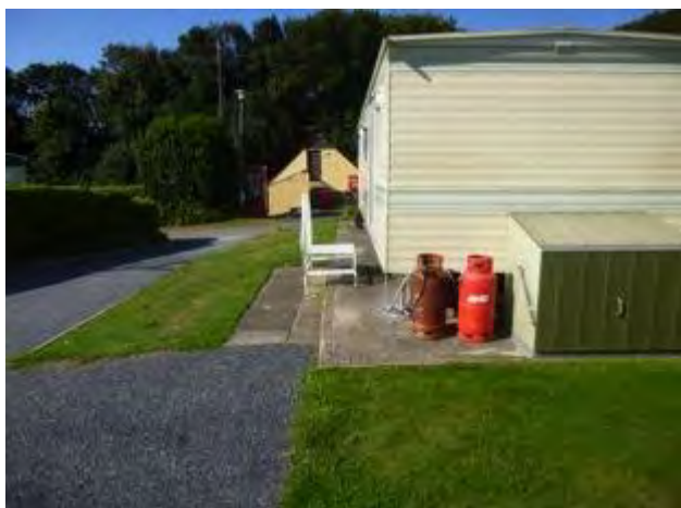
Uneven base at entrance 8
