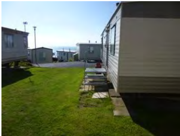
Uneven base at entrance 9
