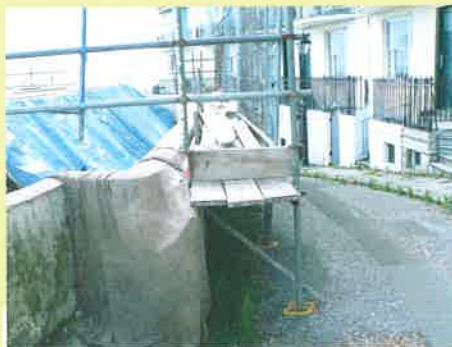
Neglected and derelict
