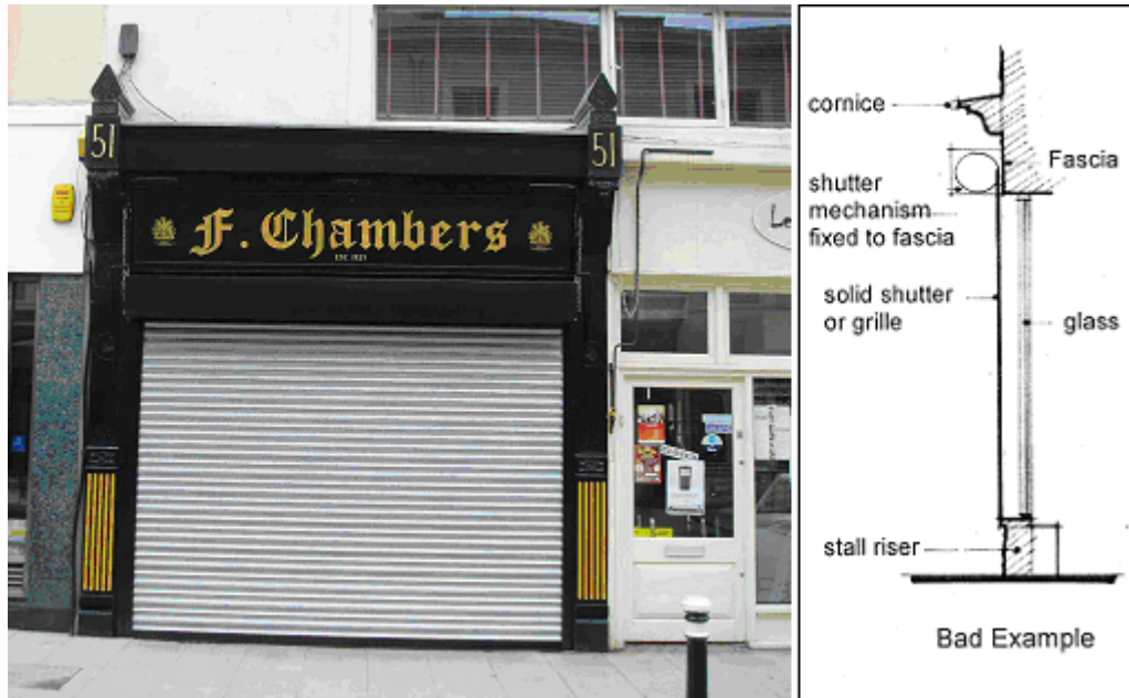
Photo showing an unacceptable 'solid' roller shutter that has been installed with the shutter box on the outside of the shopfront, masking architectural detail
